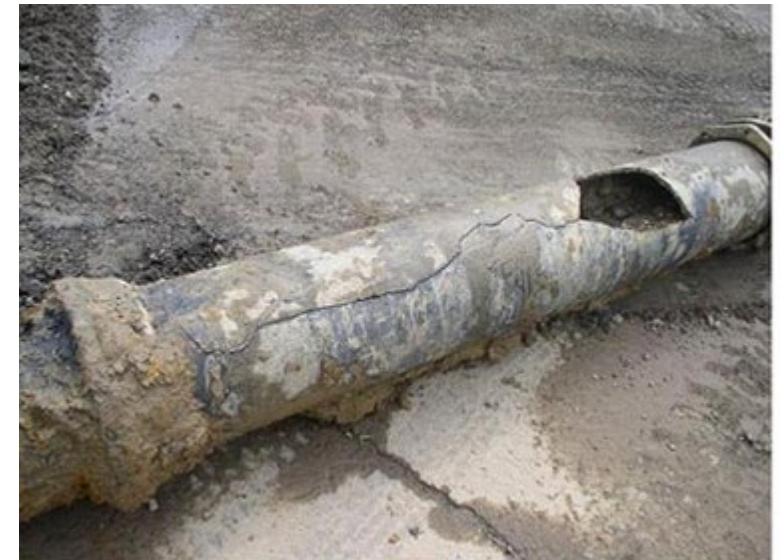
Cast Iron Pipe Broken from Water Hammer
