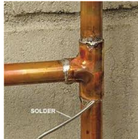
Lead Solder at Pipe Joints
