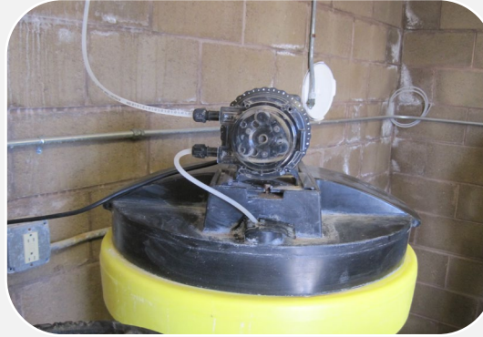
Disinfecting Drinking Water
