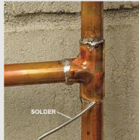
Lead Solder at Pipe Joints
