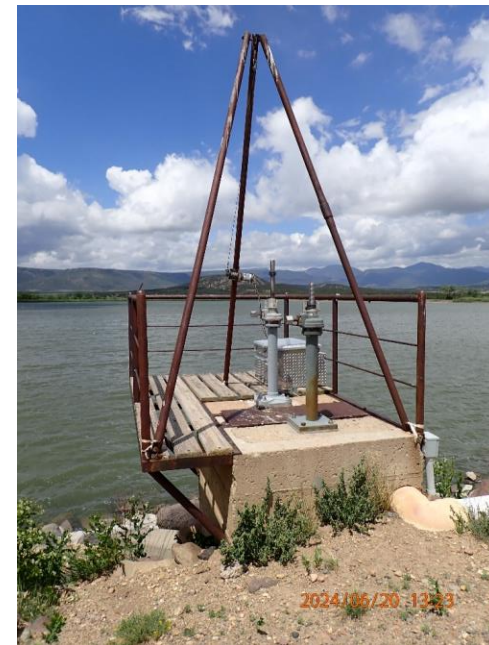
Miami, NM Lake Raw Water Intake
