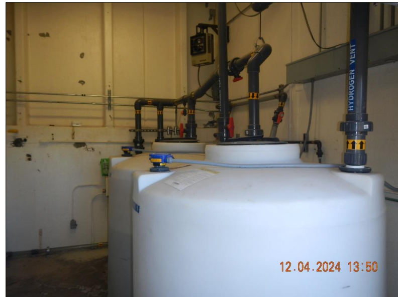
Photograph from Albuquerque Water System
