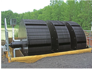
Rotating Biological Reactor “RBC”
