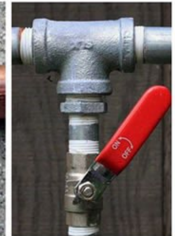
Galvanized Steel & valve
